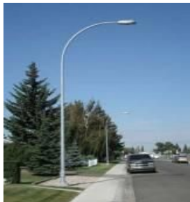
NO UPGRADE STANDARD STREET LIGHT
